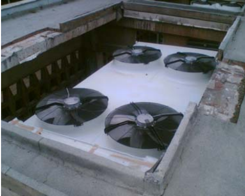
Fig. 2: Each of the condensers is equipped with 4 ebmpapst EC fans
