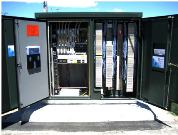
Vodafone, Orcon slam ComCom ruling on telecom cabinets (Courtesy of National Business Review 26 July 2011)
